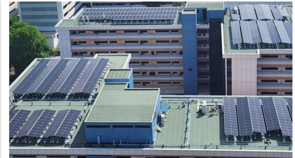
Solar panel installations on the rooftop of Kallang Basin 4 Cluster
